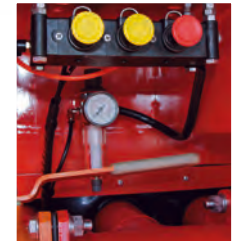
Pneumatic controls of bottom valve
