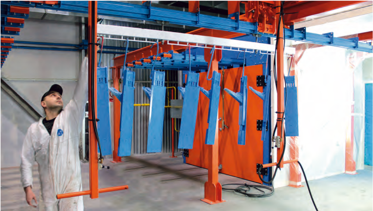
Painting line with overhead conveyor
